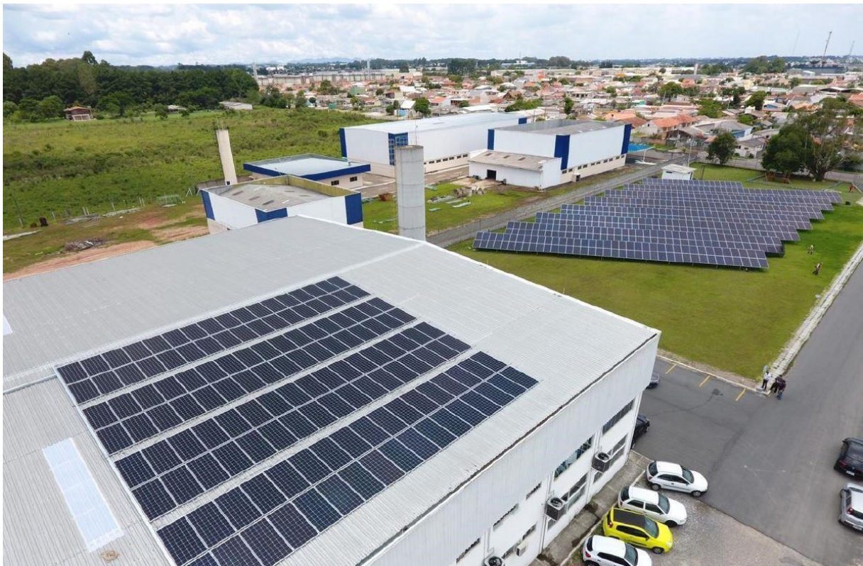
Figure 1 : Power plant at DIAM BRAZIL
